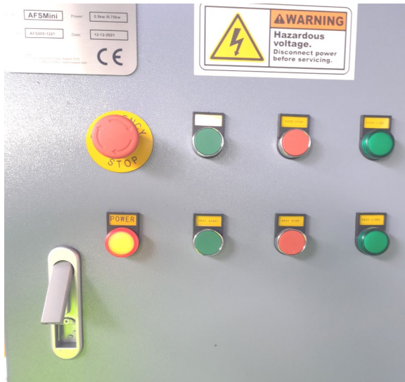
MAIN CONTROL PANEL. fig 1.
